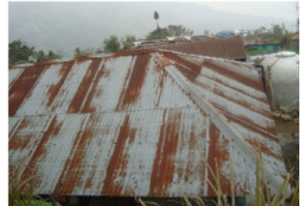
Figure 3: Rusted catchment area
