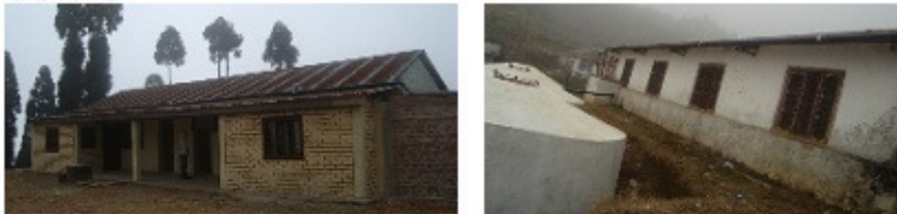
Rain water Harvesting system
