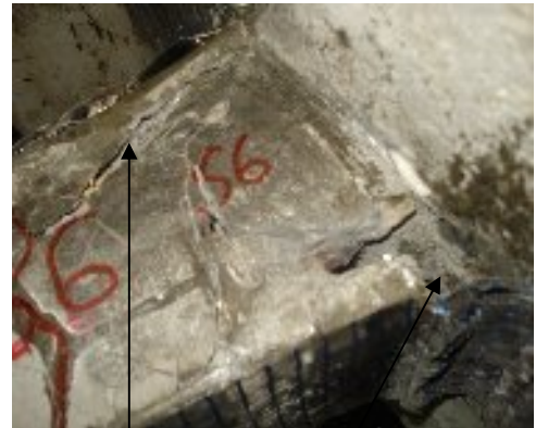
concrete crushing, delaminating of CFRP.
