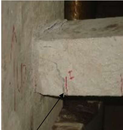
Widening of flexural crack Specimen, S8
