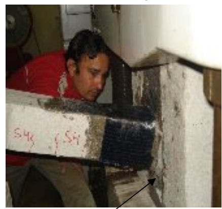
Delaminating of CFRP.
