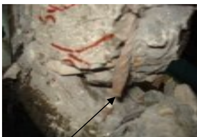
Rupture of Longitudinal Reinforcement.
