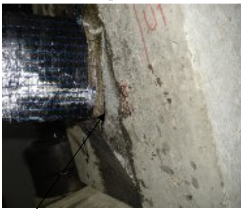
Crack at joint.
