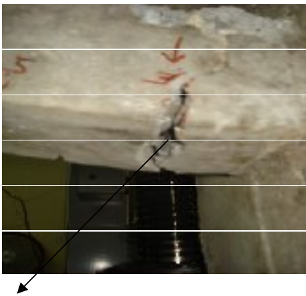
Flexural crack near interface and Concrete spalling at top. Specimen, S3
