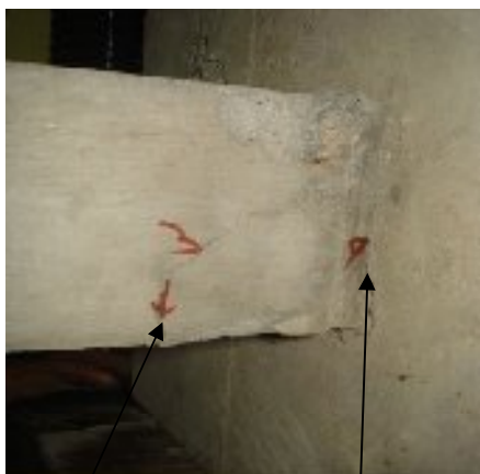
Progression of Flexural crack. Specimen, S2 Crack at joint.
