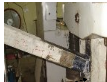
delaminating of CFRP
