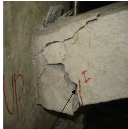
Development of plastic hinge Crushing and spalling of Concrete at corner. Specimen, S8
