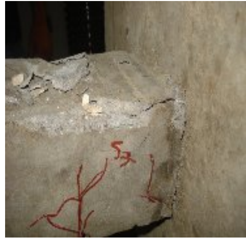
Crushing and spalling of concrete at corner and joint crack. Specimen, S7
