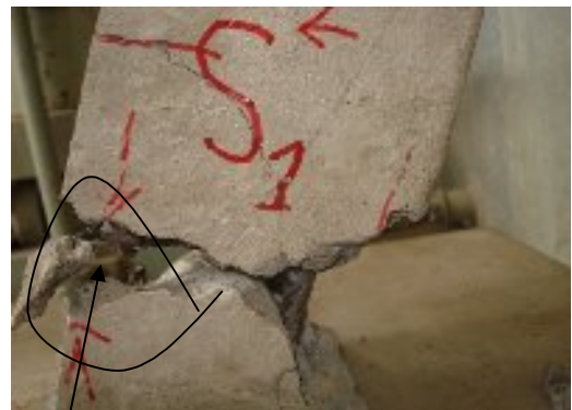
Rupture of reinforcement
