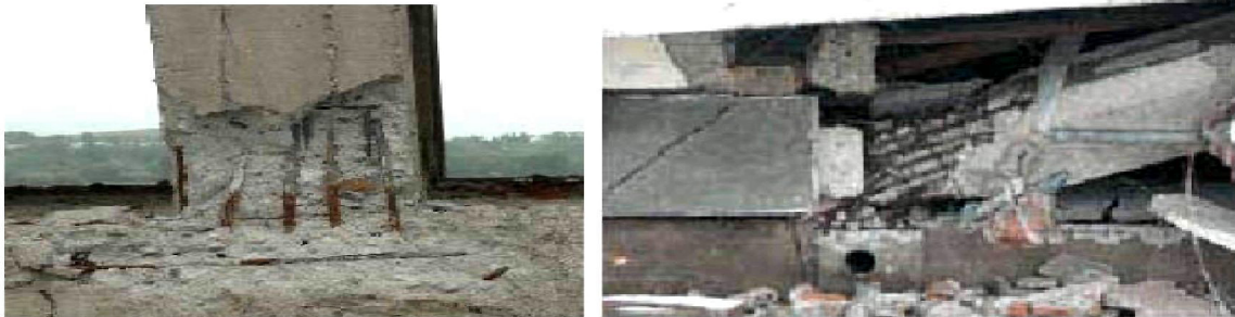
Figure 2.7: (a) Plastic hinge formation at column end during Turkey Earthquake, 2003, and (b) Lap splice failure during Sumatra Earthquake, 2004
