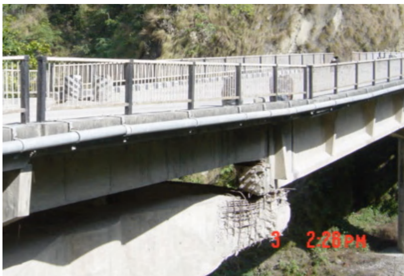
Fig. 1.2 Damage at support
