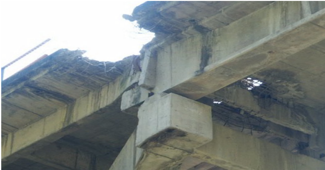
Fig. 1.1 Damage due to Bomb Blast
