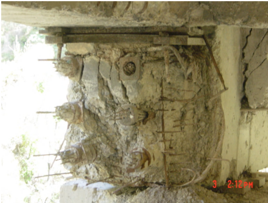
Fig.4.1 Showing damaged tendon P3, P5
