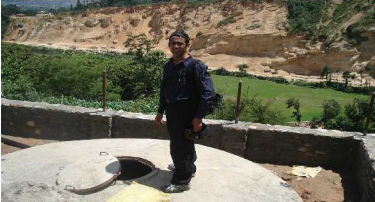
Photo - 5: Photograph of collection chamber of drinking water in under-construction position observed by researcher while collecting data
