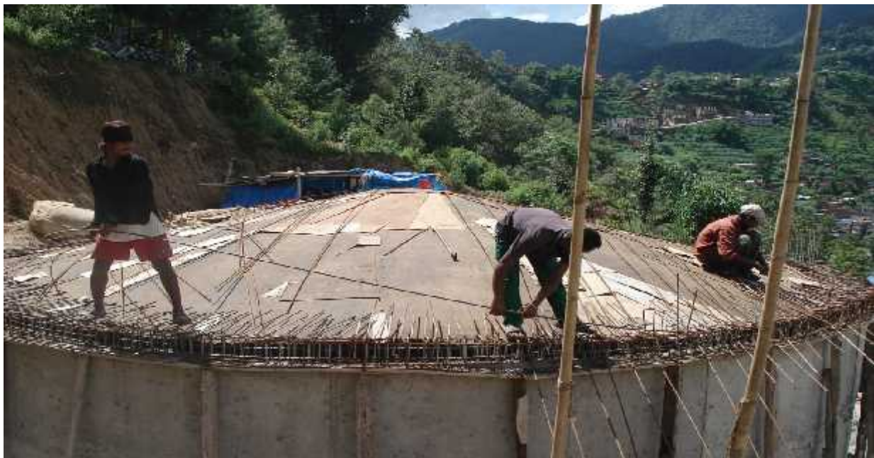
Photo – 6: Photograph of collection chamber of community managed drinking water in under-construction position
