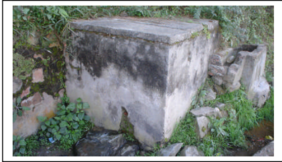
Well Tank, Ward No. 13
