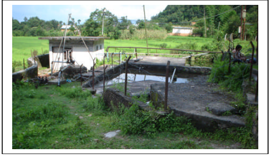
Under Ground Spring & Reservoir, Ward No.7
