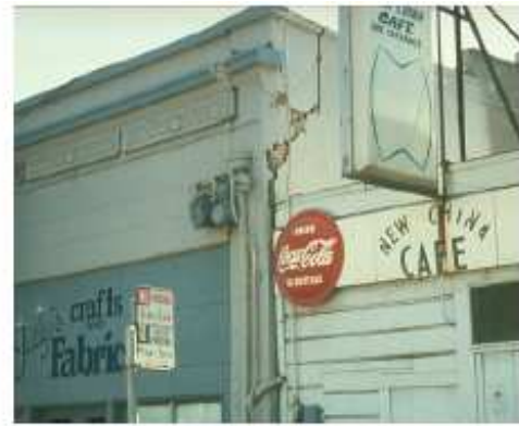
Hollister Area, Loma Prieta Earthquake, 1989
