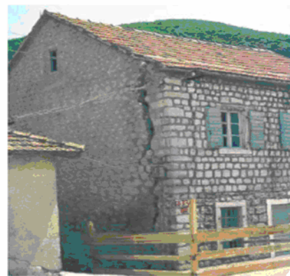
Figure 2.6 Separation of wall corner
