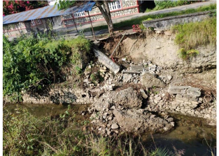
Photo 2: Structural damages at Main Canal
