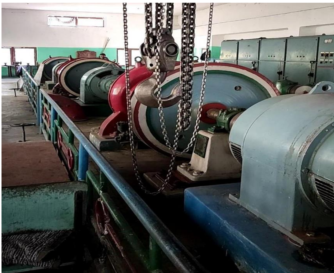
Figure 3: Turbine-generator units at Powerhouse
