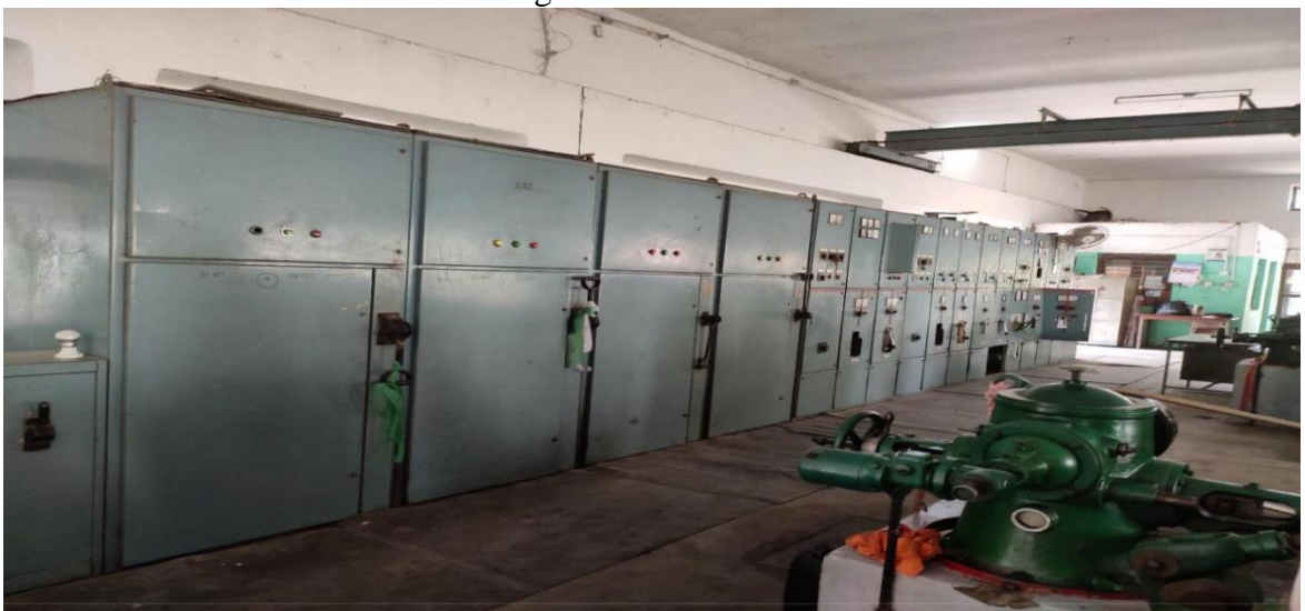
Photo 8: 11 kV Switchgear Panels
