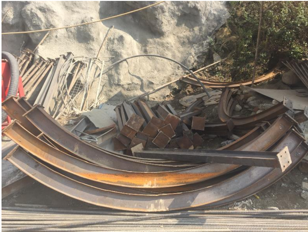
I-Beam Used as the Rock Support Sample from Site
