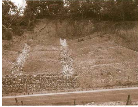
Figure 16: Stone-pitched surface drains on a wet landslide scar
