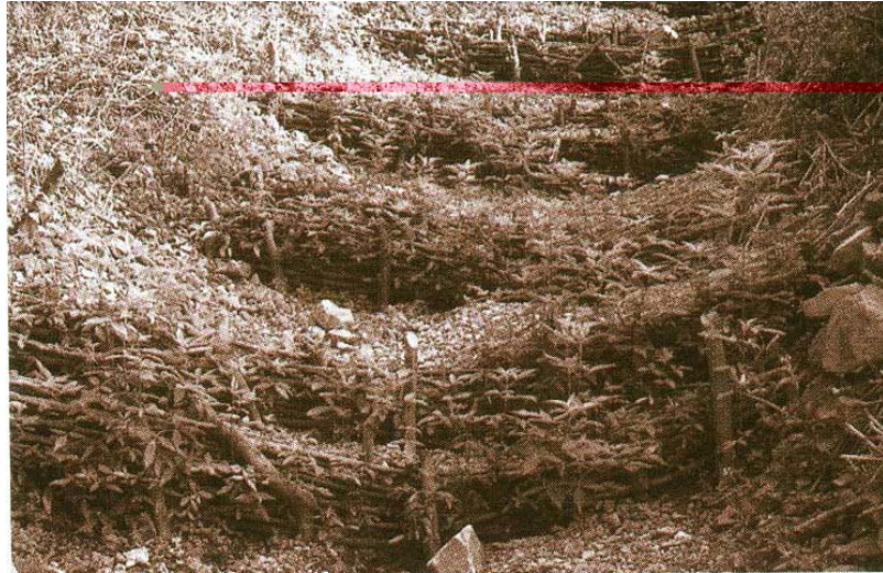
Figure 8: Live check dams form a strong barrier on a wide range of gully sites, on slopes up to 45^{\circ} .
