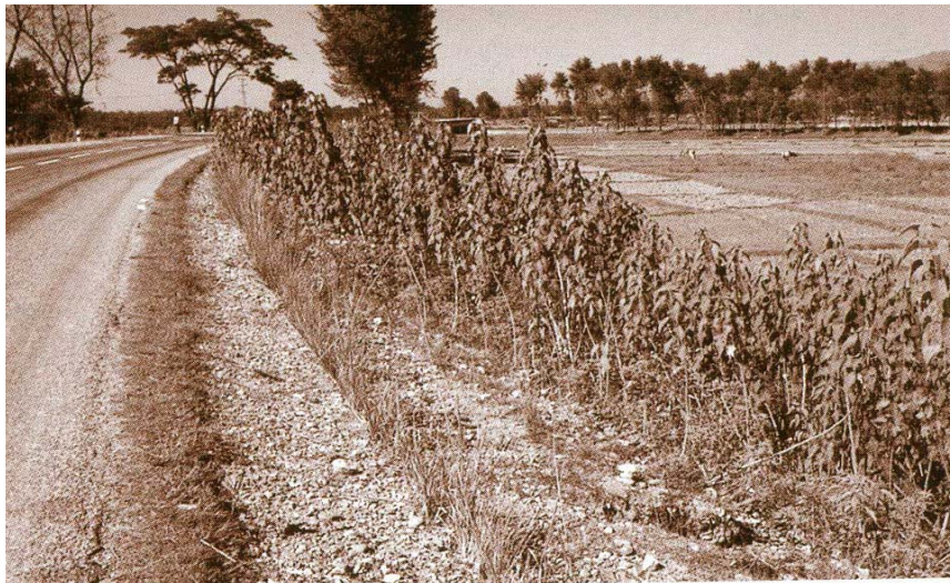
Figure 3: Turfing- It provides instant surface protection, as used on this road shoulder (the embankment has been treated with grass lines and brush layering).
