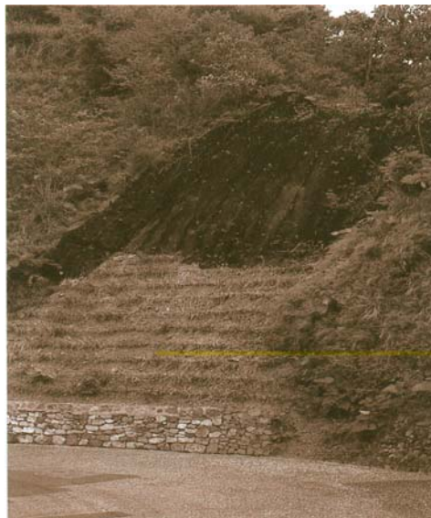
Figure 13: A revetment toe wall, protected by grasses planted on the slope
