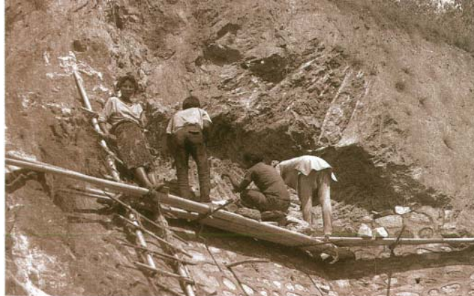
Figure 14: Construction of Cement masonry dentition wall to prevent undercutting of the upper part of a steep cut slope in differentially weathered gneiss.
