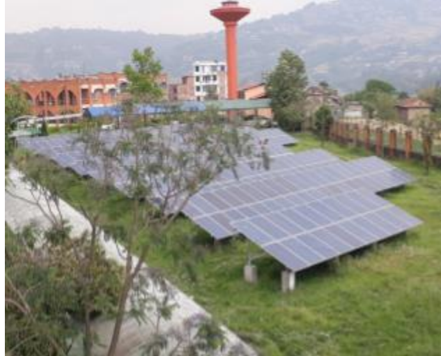
Figure 2-24: Grid-Tied Solar Power Plant at Kharipati (Tiwari, 2017)
