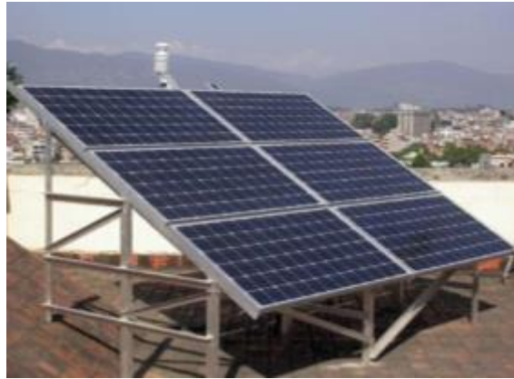
Figure 2-26: Grid-Tied Solar Power Plant at CES (Bhattarai, 2013)
