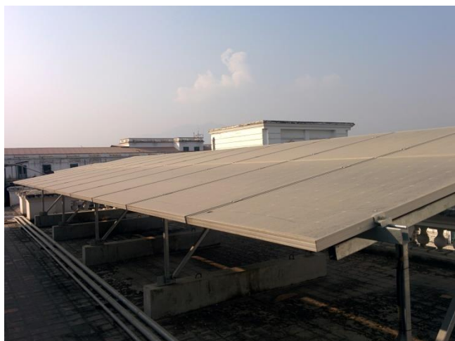
Figure 2-25: Grid-Tied Solar Power Plant at Singha Durbar
