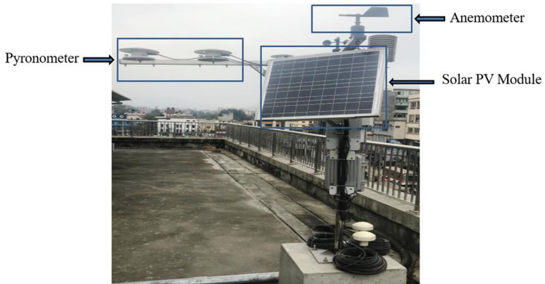
Figure 1-2 Measuring instrument connected on the rooftop of the K3 substation.
