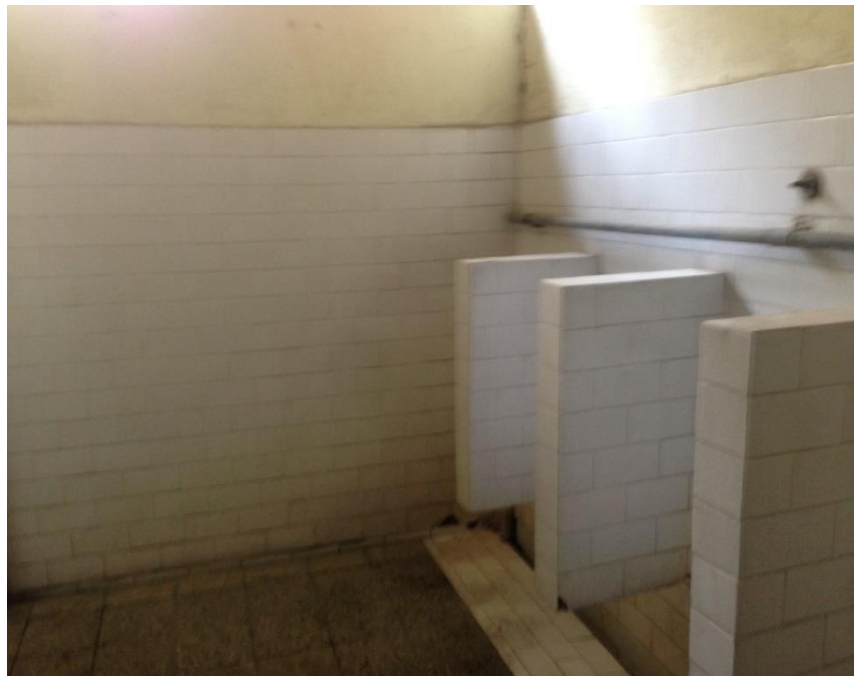
P2: Existing urinals at Pulchowk Campus
