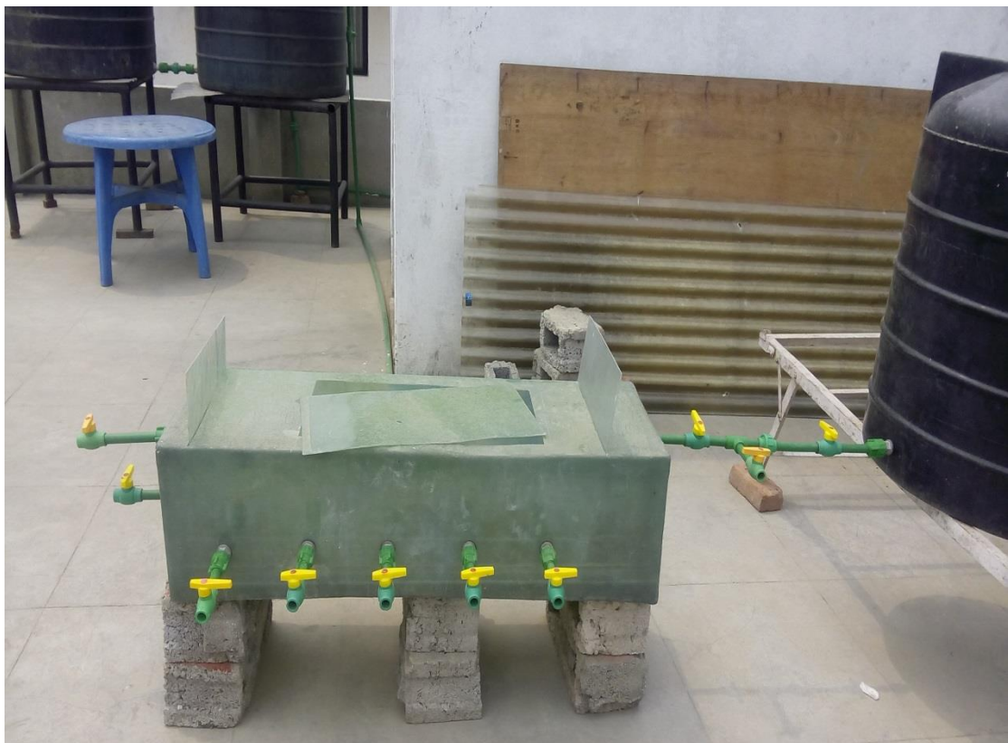
P6: Sedimentation tank
