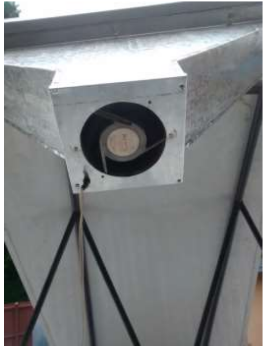
Blower Fitted in Duct
