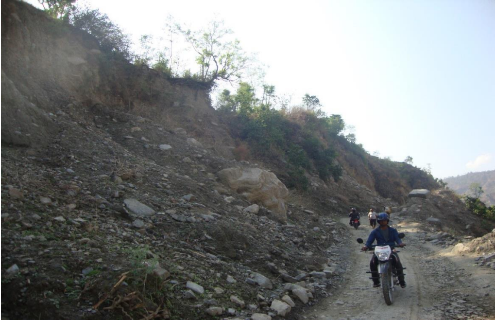
Figure 0.4 Landslide view which is on the Right bank of Sunkoshi river at Ghurmi Bridge
