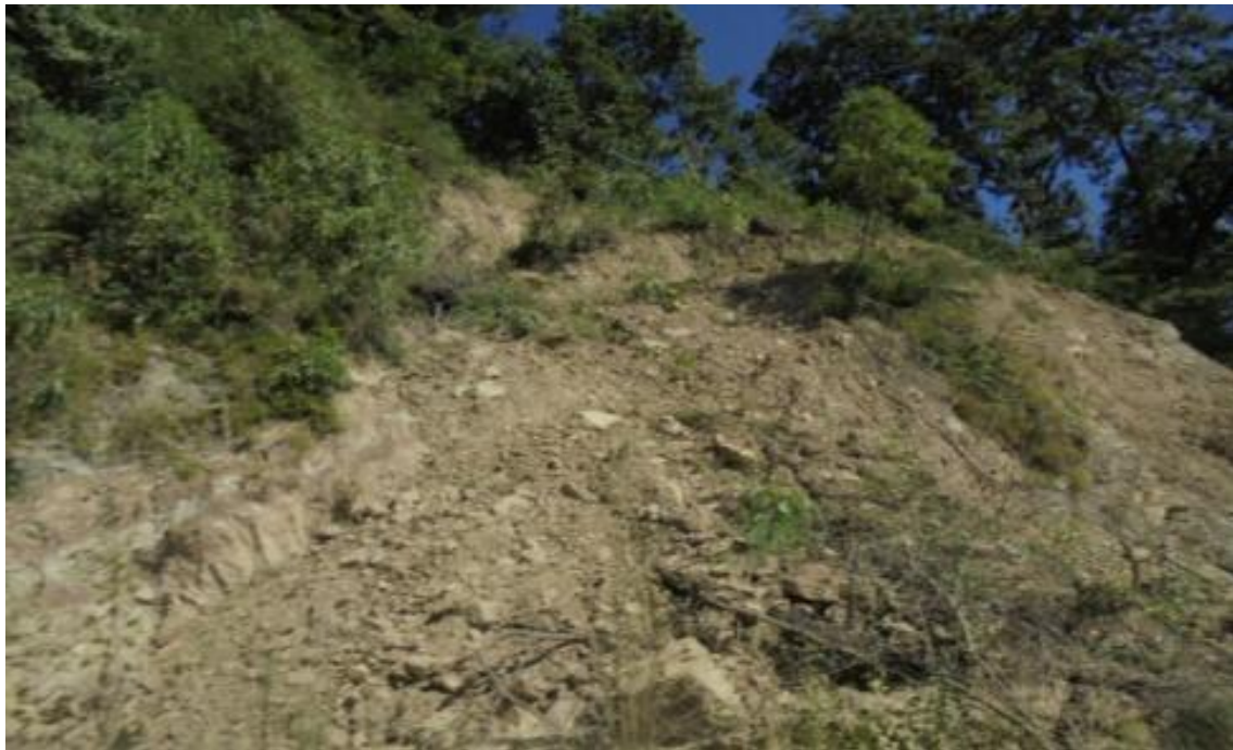
Photograph 6. Landslide observed near Shreepur Chhatiwan in the watershed.
