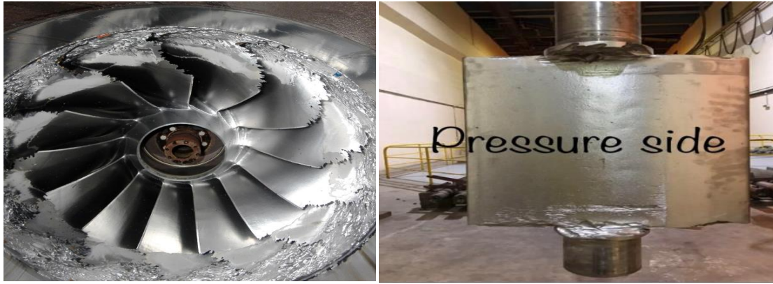
Figure 1.1: Eroded runner and guide vane of Kaligandaki HPS obtained during site visit
