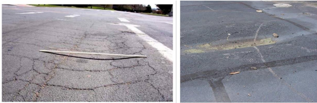
Figure 1.1 Subgrade Rutting in Flexible Pavement
