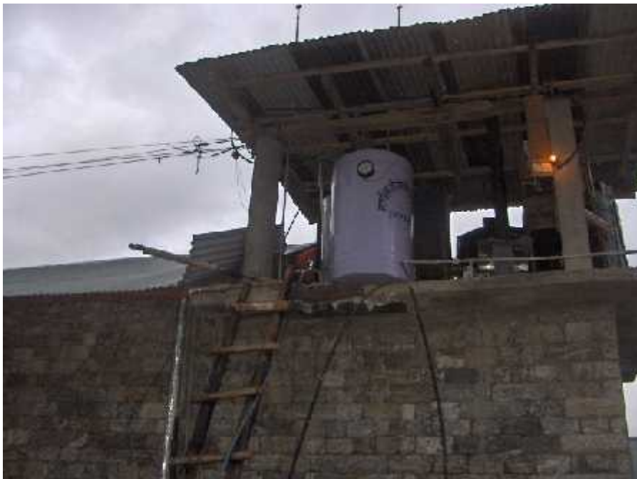
A kerosene water boiler being used by the Mera Lodge at Lukla. As of May, 2006, there were only three such water boilers in Lukla.
