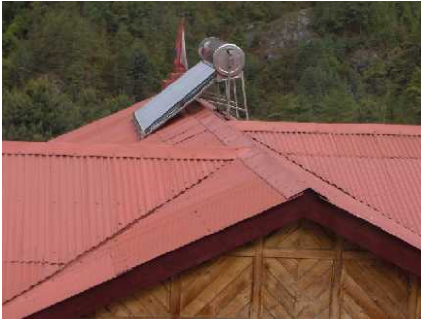
A solar panel installed on top of the Everest Summit Lodges, a posh lodge at Monjo.
