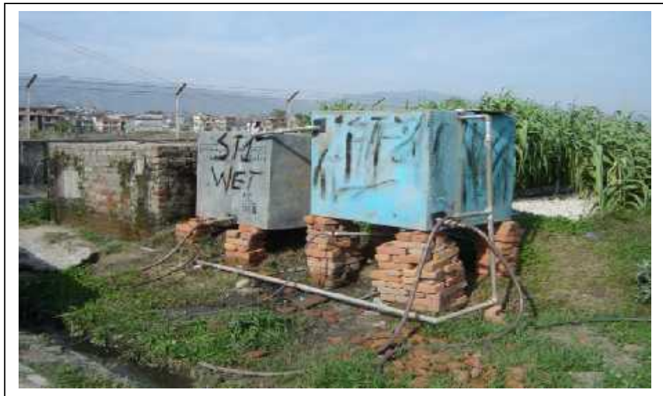
Photo 2: Settling tanks for pre-treatment.
