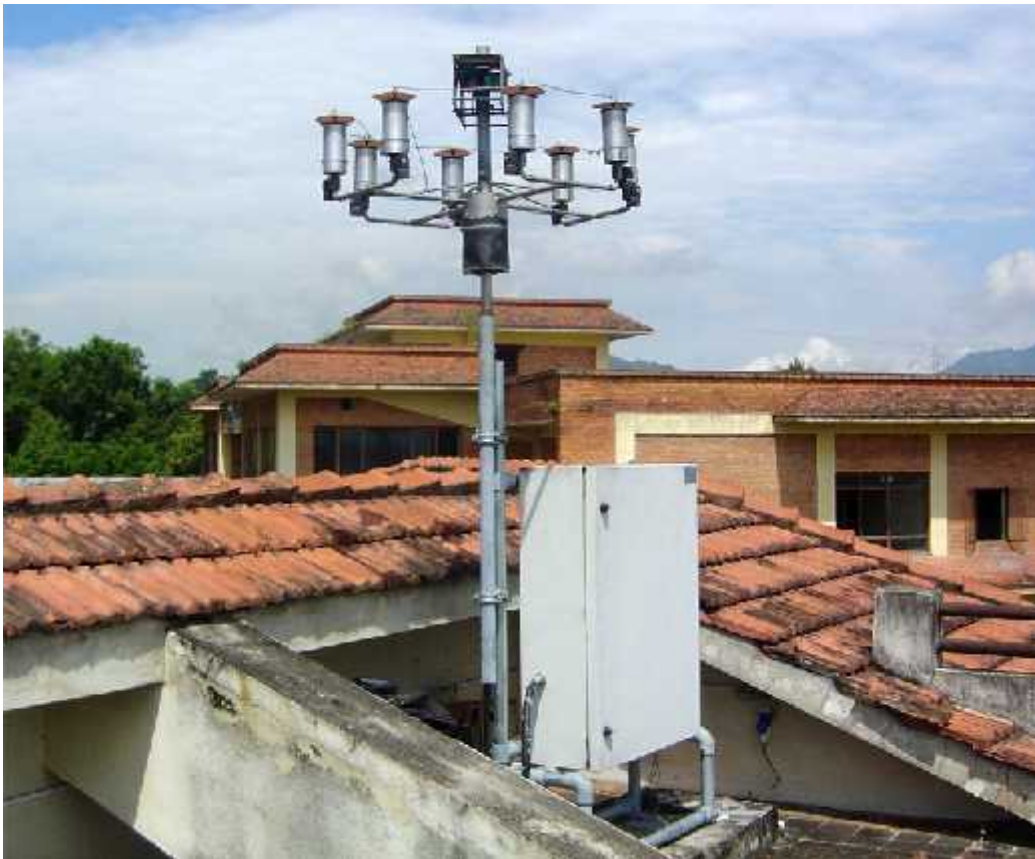
A Sample of Air Quality Monitoring Station located at TU, Kirtipur
