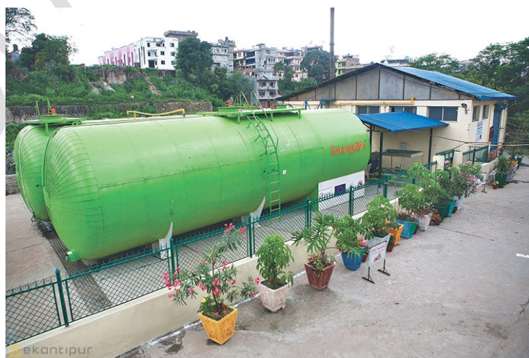
Figure 6: Energy Plant at Teku Collection Center (Source: Internet)
