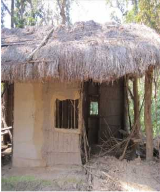
House damaged by wild elephant
