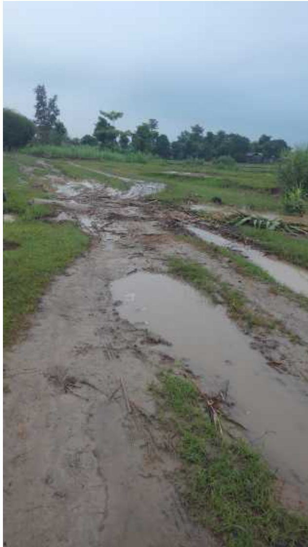
Photo 3 : Flood Destroyed the Road
