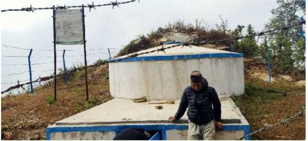
Photograph of Water Tank Constructed by the Program
