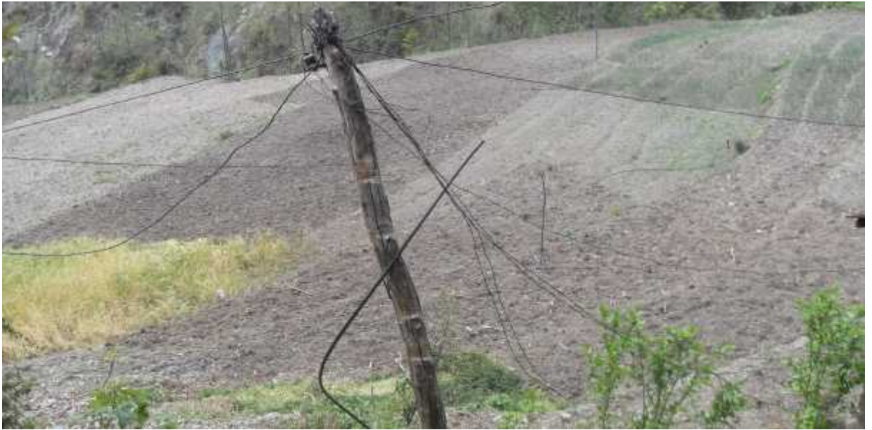
Photo 7: Electricity distribution pole and lines.
