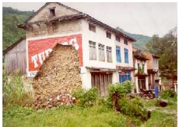
Earthquake in Dhading 2045 BS
