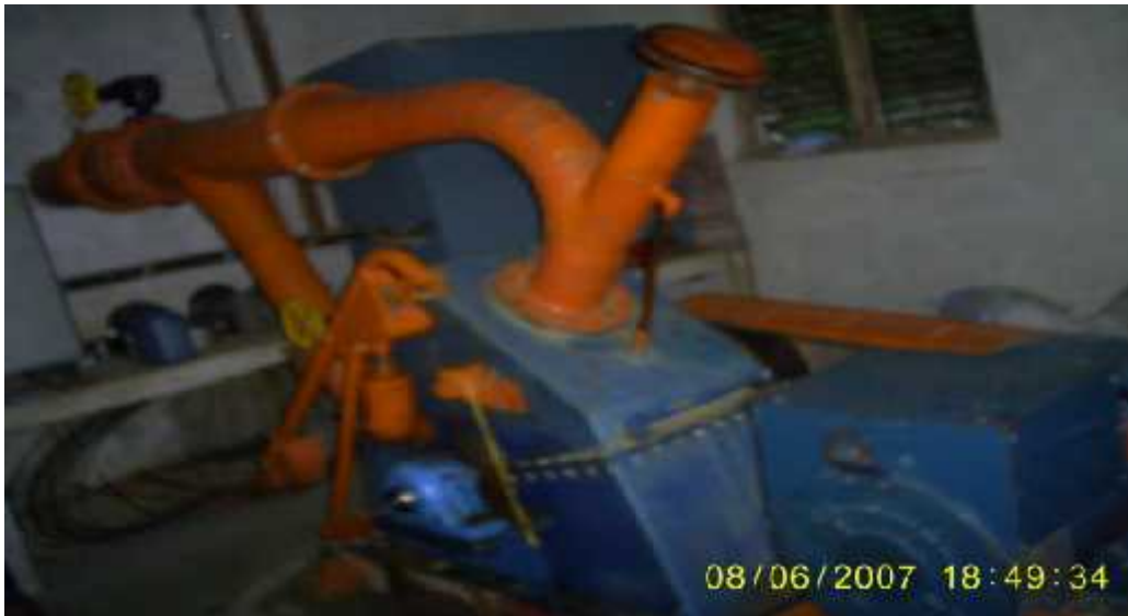
Turbine of the project
