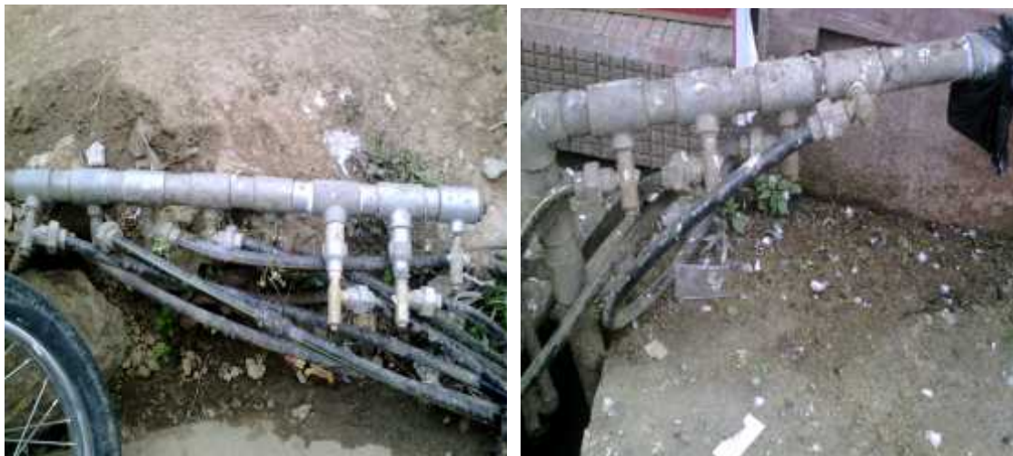
Photo 5.2: Pipeline in Ilam Municipality
