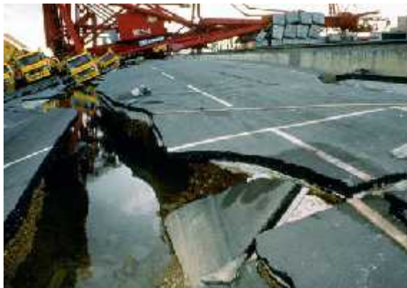
Photo 2.3.1B.: Road structure Collapse, Kobe Japan
