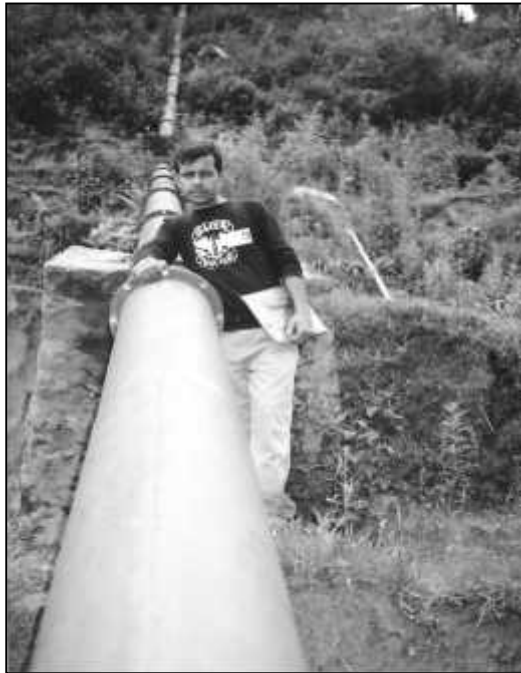
Penstock Pipe of MHP
