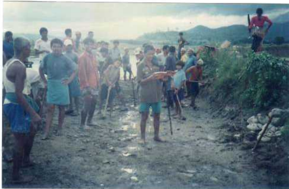
Photograph 4: Checking attendance of 'Kulo' owners by Metha with measuring bamboo stick during repairing time.
