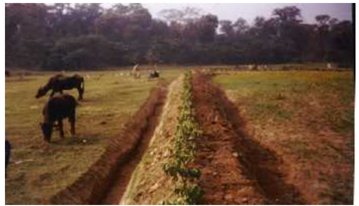
14. Trench made by local people to remedy from crop damage
