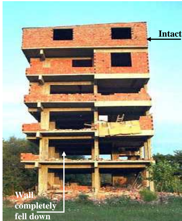
Damage to Infill wall only in Gölcük Fig-A3
