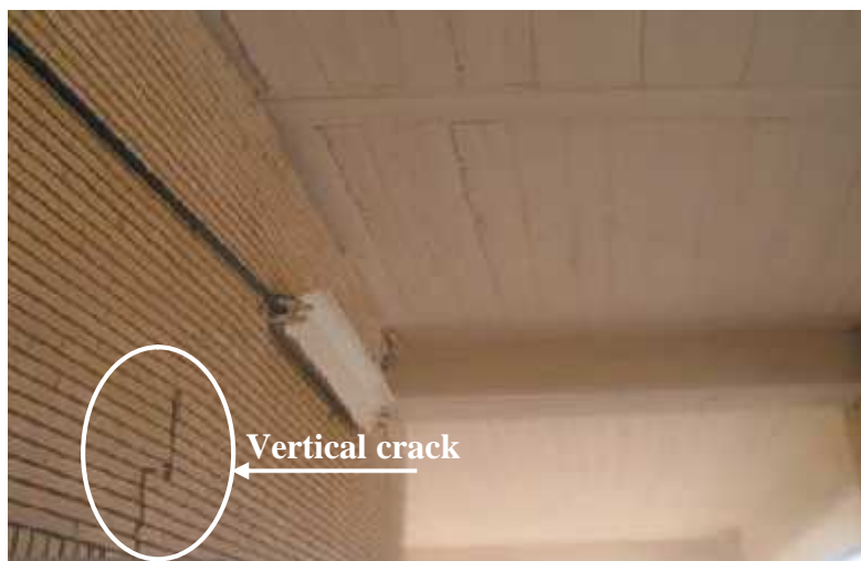
Wall shearing tendency to fail in orthogonal direction (Bam, Iran)
